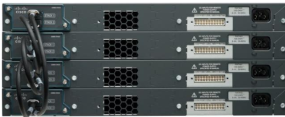
Figure 3. Cisco FlexStack Module and Switches
